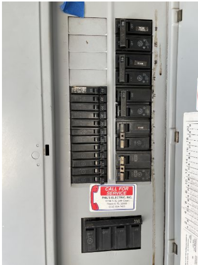
200 amp GE electrical panel
