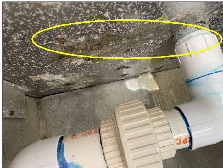
Several areas had water coming down and filling up the bottom of the enclosure. Recommend a licensed contractor for evaluation and repair as needed.
