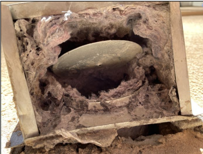
View of dryer vent coming out of the back of the house. Recommend cleaning.
