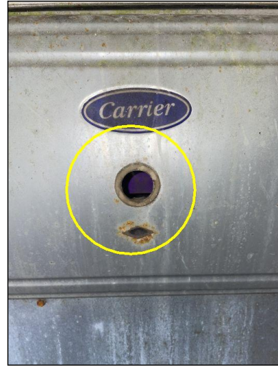
There was a hole on the front cover to the air filter compartment, this is continually sucking in outside air from the garage. Recommend sealing it up.
