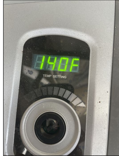
Tankless water heater was set to 140 degrees. This is considered a scalding temperature to the skin, and can also overwork the heating element prematurely.
