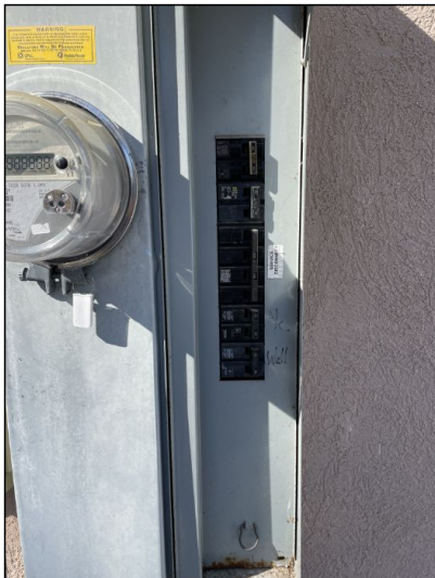
200 amp Siemens electric main panel outside of the garage.
