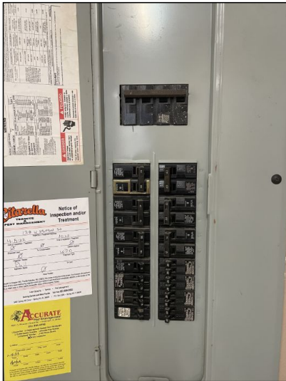
200 amp Siemens electric secondary panel in the laundry room.
