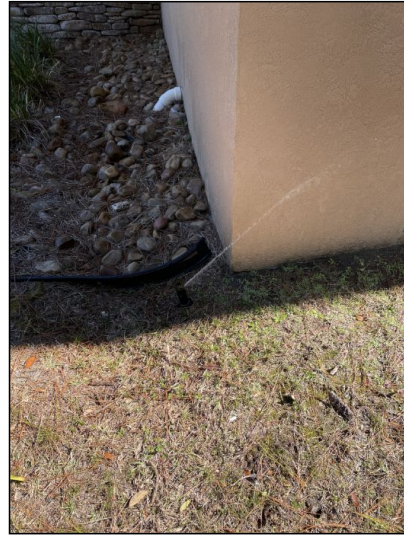
Sprinkler system needs adjustment, heads were spraying the house and into other areas not designed to be watered.
