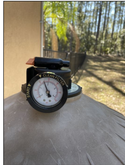
Picture of the pool filter pressure gauge. Pressure gauge was reading high and in the warning zone to clean the filter.
