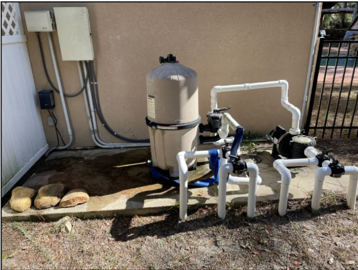
Pool filter, pump. The system was running and electrically bonded as required.
