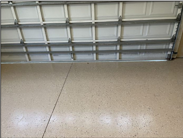
The garage door did not seal all the way when closed, needs adjustment.
