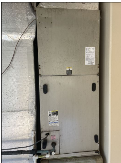
Air handler, Carrier, model from 2010. 10 KW heating strip in unit.
