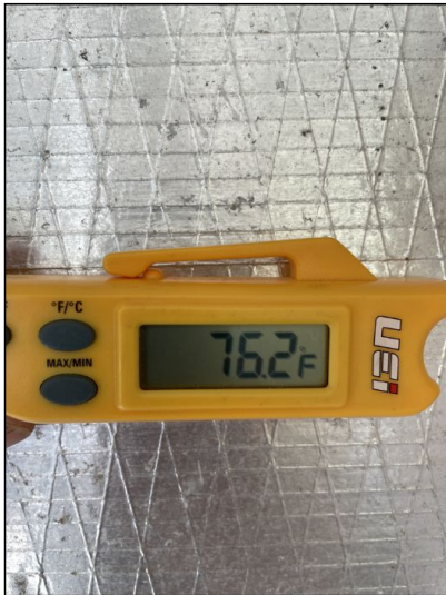
Pic of the air being taken back in at return. 26 degree split.
