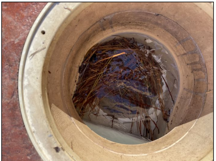
Skimmer was full of debris.
