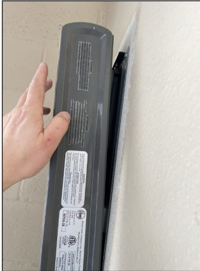
The tankless water heater enclosure was loose on the wall.
