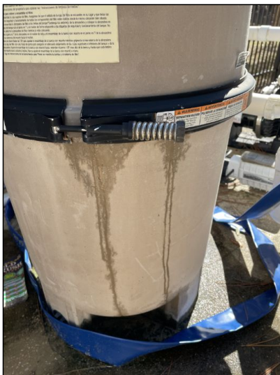
Water appeared to be coming out of the filter on the day of inspection. Recommend a licensed pool technician for maintenance on the system.
