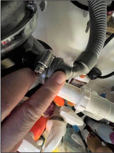
There was a kink in the dishwasher drain hose/food disposal connection under the kitchen sink. Could impede water flow.
