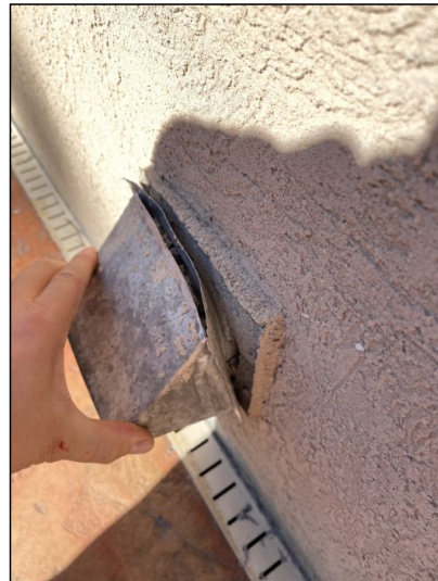
Dryer vent connection was loose on the house.
