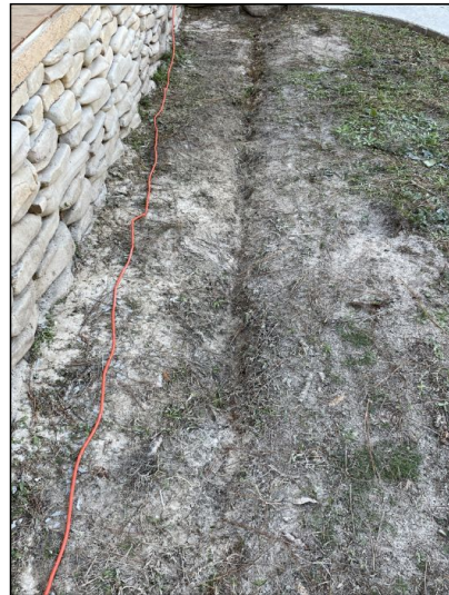
Minimal erosion due to not having gutters and down spouts.
