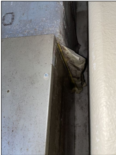
Loose tape around the top of the air handler/trunk connection. Recommend maintenance.
