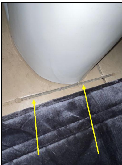
Grout missing in front of the master bathroom toilet.
