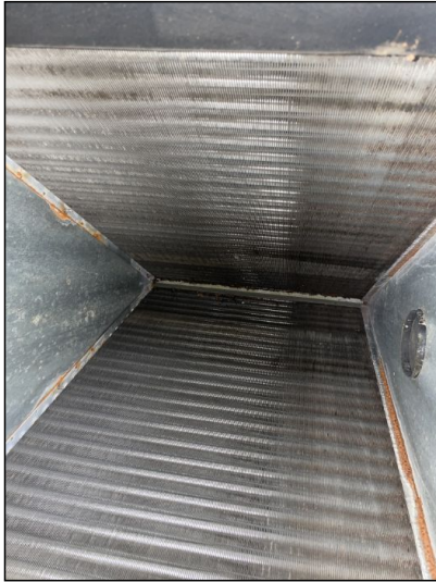
View up the air handler at the evaporator coils. Small amount of rust forming on the outside coils, overall satisfactory.
