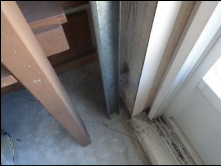
There is no safety reverse on the garage door.
