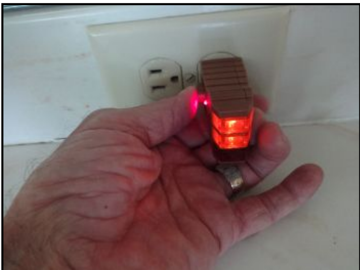
There is no GFI protection in the bathrooms of this home.
