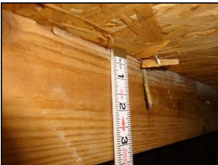
Hurricane nailing in the attic, good for Wind Mitigation deduction on Homeowner's.
