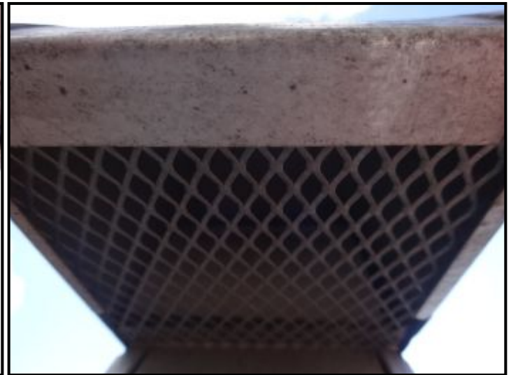
While this is to the bathroom vent, this is what the previous dryer vent should look like for better efficiency.
