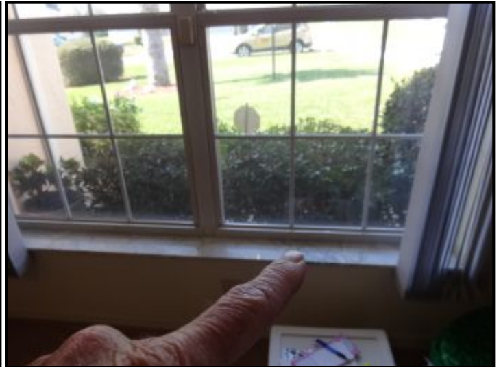
There are two windows with broken plastic on them. This one is the right front window, in the living area.
