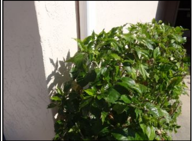
Vegetation up against the home, recommend trimming back some.
