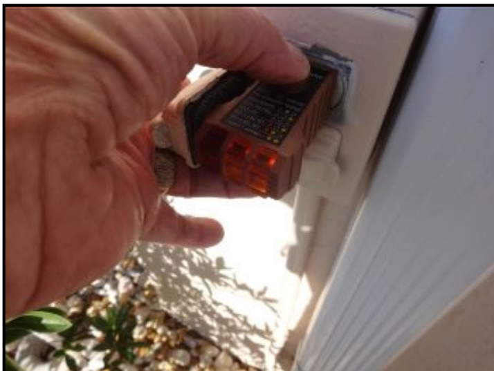
There is no GFI protection on the exterior of this home.
