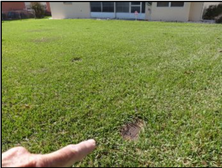
Water shutoff in the meter box in back of the home.
