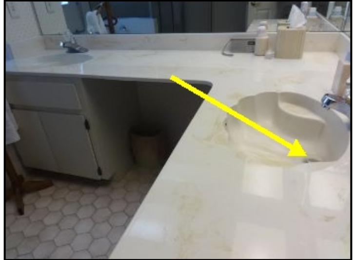
In the master bathroom, the sink stopper in the right sink does not hold water.
