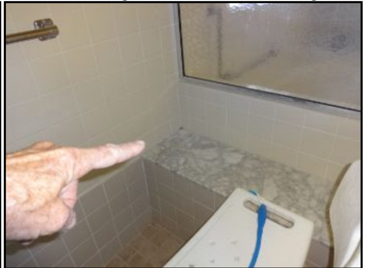
Recommend caulk around the main bathroom shower tile.
