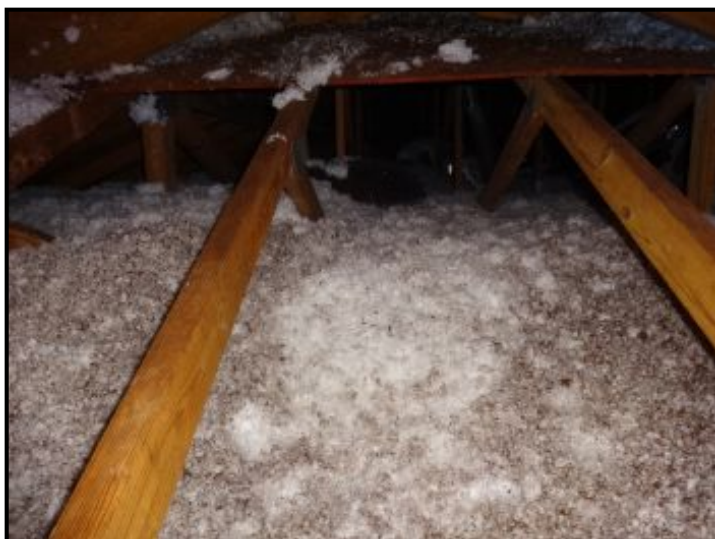
Loose insulation depth measurement, over 10 inch average, R 30.
