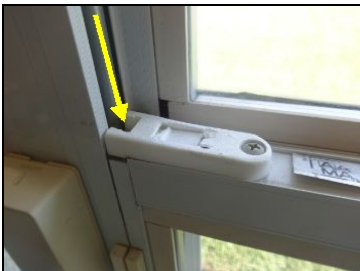
The broken clip from the previous window photo.
