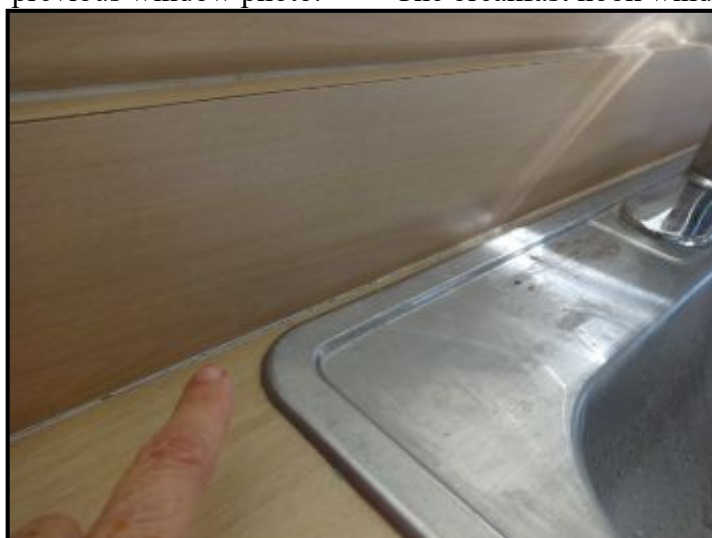
Recommend caulk around the kitchen sink counter/backsplash.
