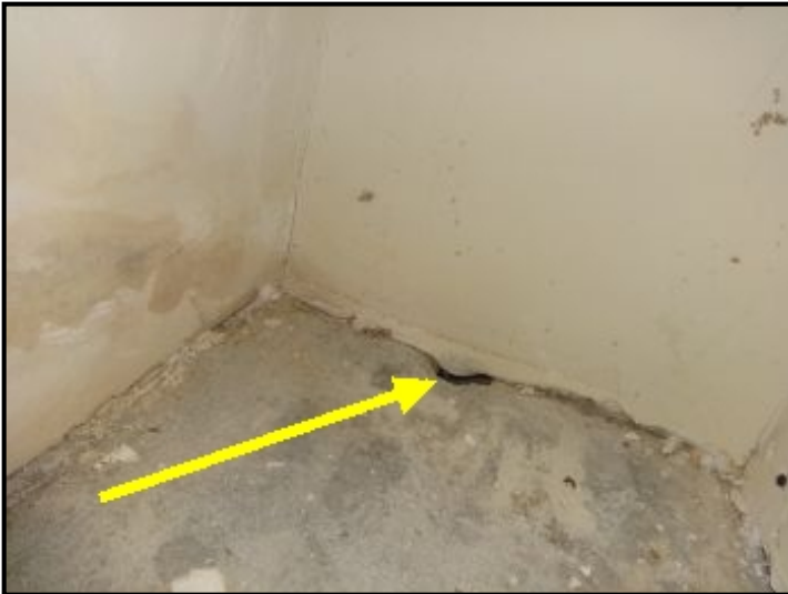
In the low cabinet in the northeast bedroom, this hole in the slab was noticed by the pest guys.
